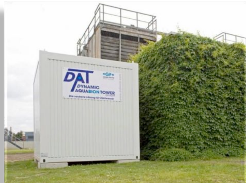
External container solution
